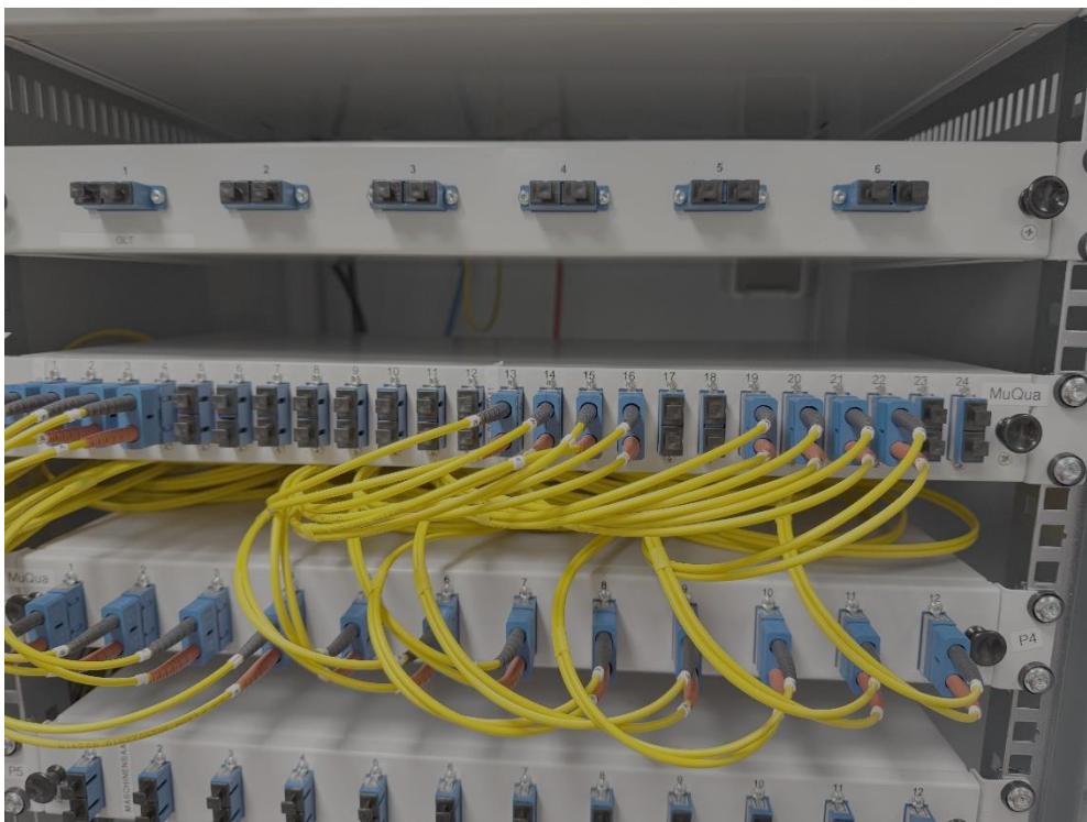
Rohde & Schwarz container patch panels
