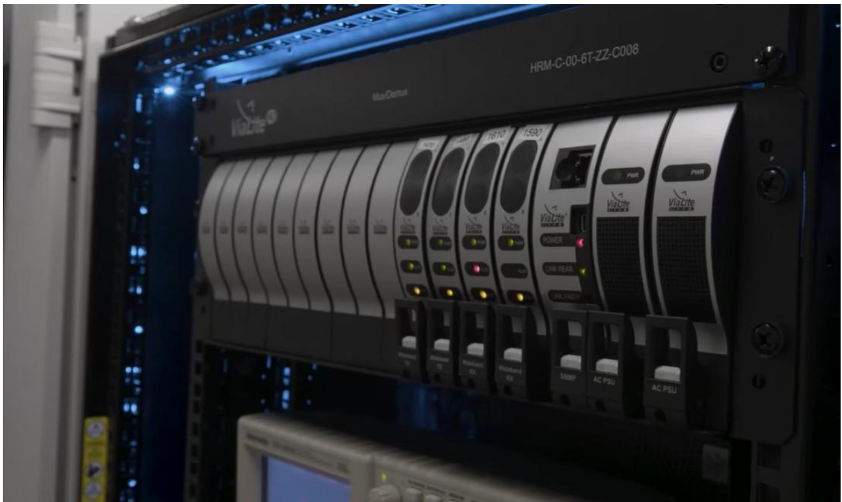
Fig. 3 Server rack at the HTW.
